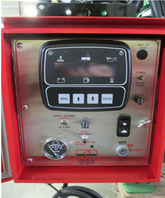
EP-3 control panel
